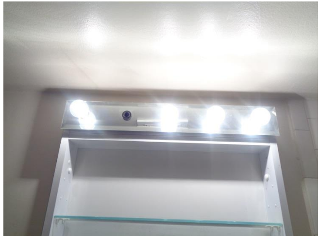
Figure 19: Typical Apartment Bathroom Fixture
