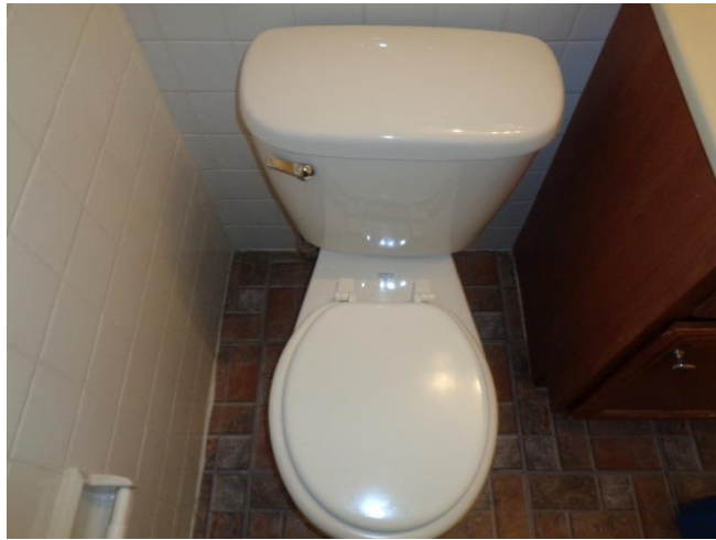
Figure 28: Typical Existing 1.6 GPF Toilet
