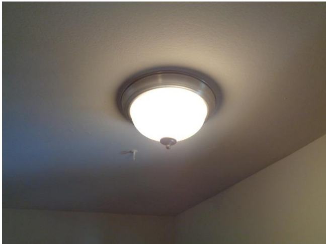
Figure 18: Typical Apartment Fixture
