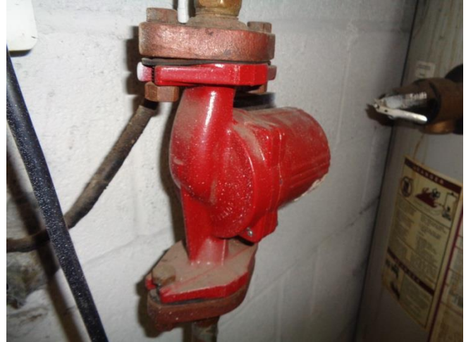
Figure 15: Typical DHW Recirculation Pump
