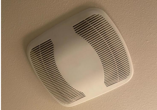
Figure 10: Typical Exhaust Fan in Apartment Bathroom
