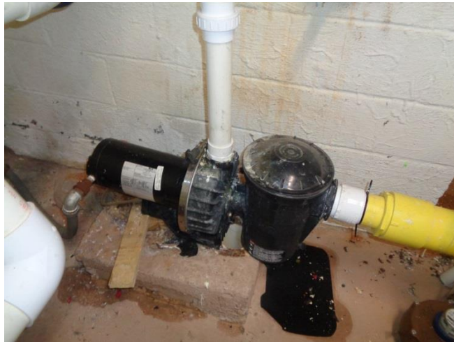
Figure 30: Existing Pool Pump
