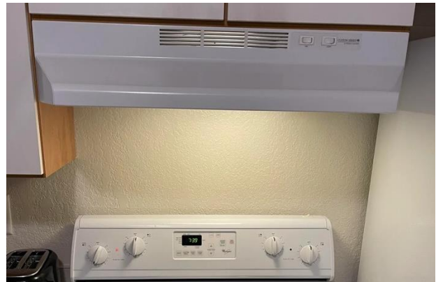
Figure 11: Typical Ductless Range Hood in Apartment Kitchen
